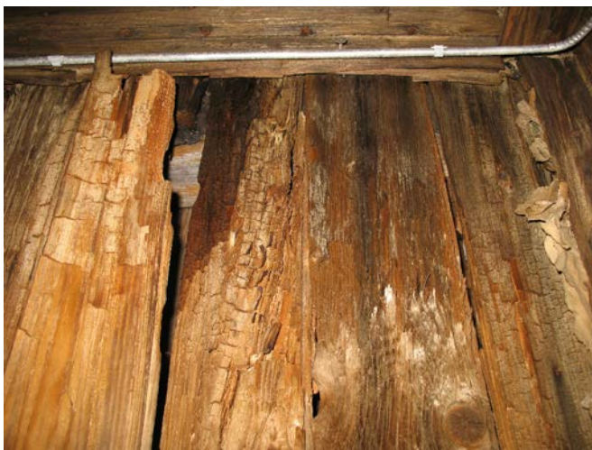
Figure 7. Extensive brownrot decay in upper part of wall caused by Leucogyrophana mollis .
