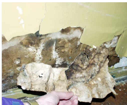
Figure 5. Extensive decay by Coniophora puteana in a water damaged wall.
